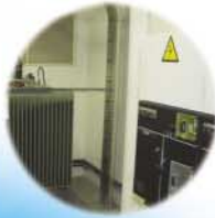
High-voltage cables for power distribution
